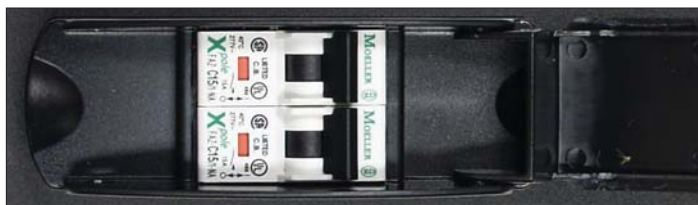
UL 489 hydraulic-magnetic circuit breaker on 30 Amp PDU.
