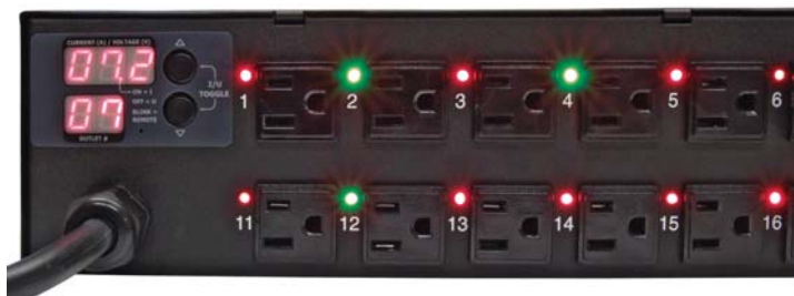
Rear of 2U PDU showing current draw for outlet #7. Red LEDs show outlets that are switched on. Green LEDs show outlets that are switched off.
